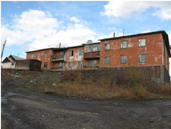
Village Udarnik, on license area, pop. seasonal, buildings in place to house miners
